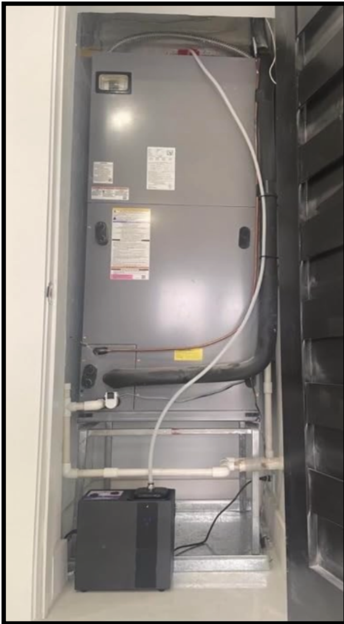
Example of diffuser tubing routed to an HVAC air-handling unit
